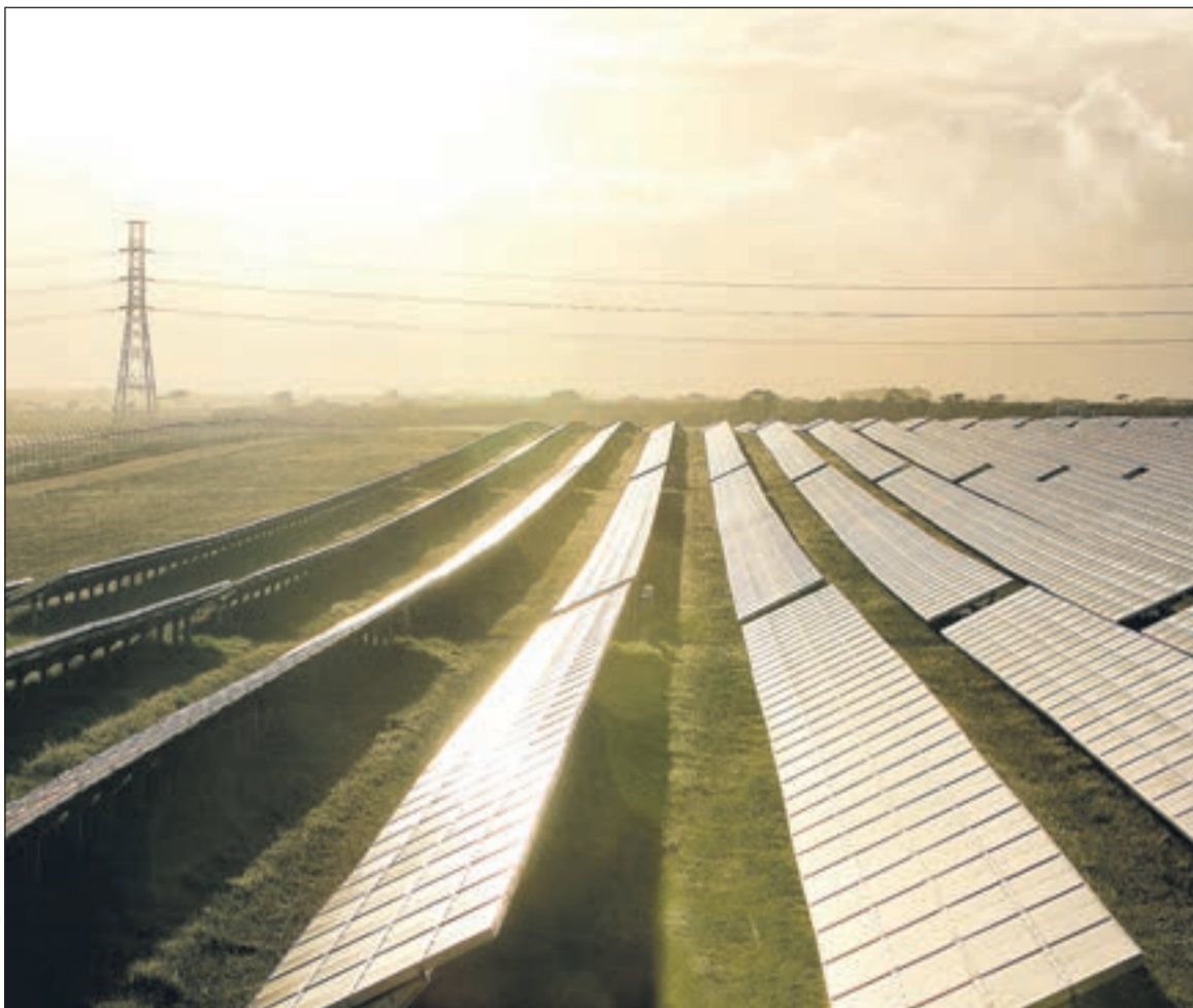
POWER PACK: The country's first utility-scale solar farm has opened near Geraldton, with 150,000 solar panels covering 50 hectares of farmland (see page 25).
